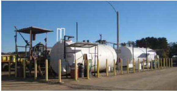
Figure 2. County Highway Garage Diesel Tanks
