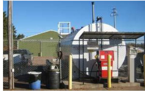
Figure 3. County Unleaded Tank
