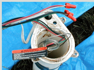
FIGURE 3 (WIRES IN WELL CASING)
